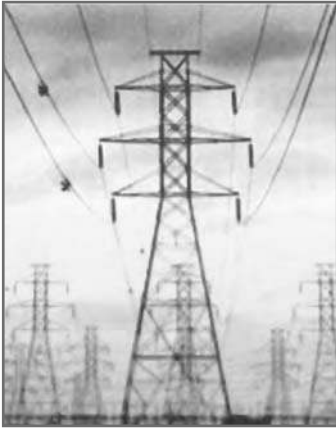
Fig. 3.9: National Power Grid to supply Electricity
