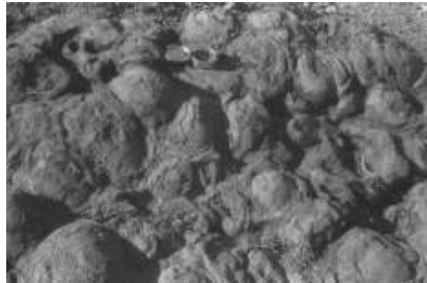
Fig.6.4 : Exfoliation (Flacking) and granular disintegration
