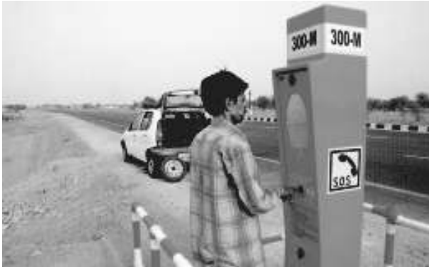
Fig. 7.10 : Emergency call box on NH-8
