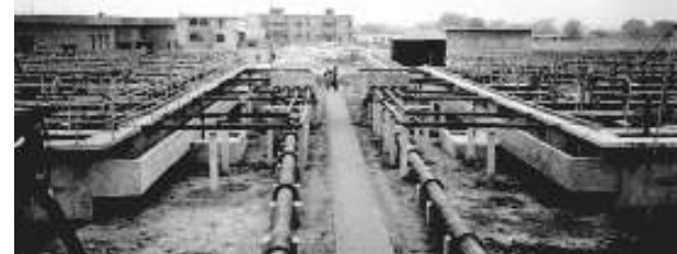
Fig. 6.11: Sewage Treatment plant under Yamuna action plan at Faridabad
